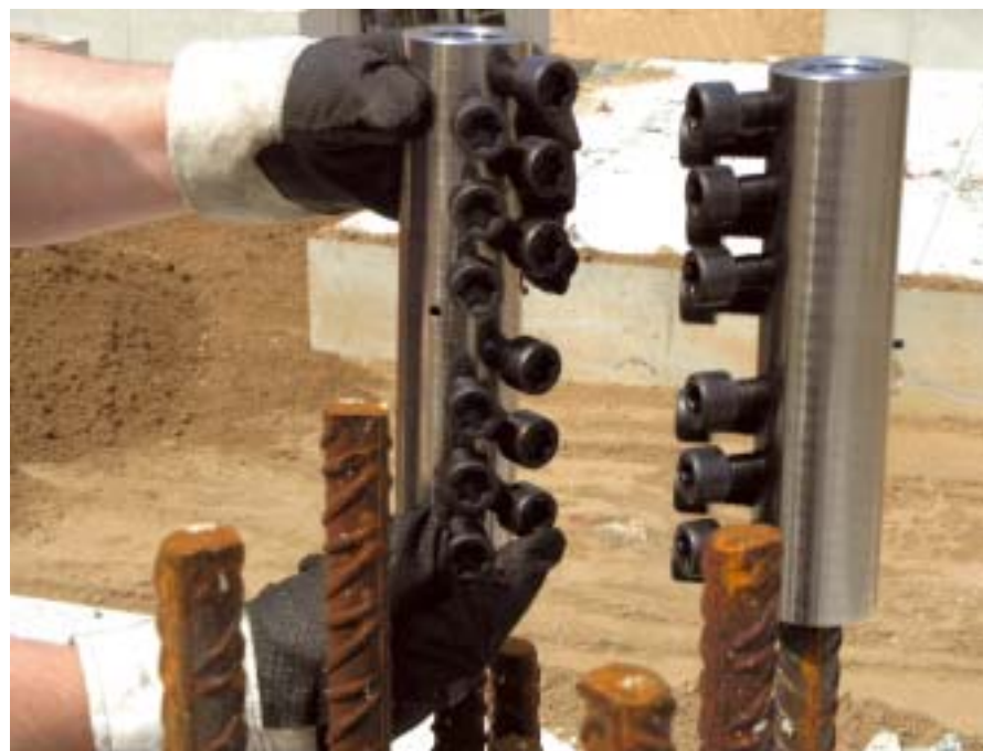
HGC coupler after installation
